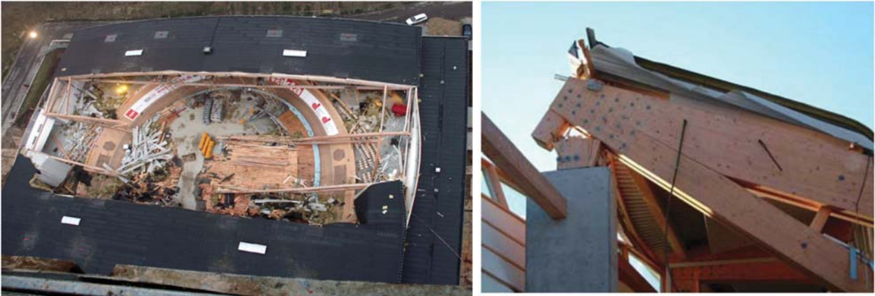
Figure 6-43 – Collapse of the timber roof of the Siemens Arena in Ballerup, Denmark (from COST Action E55, 2010)
