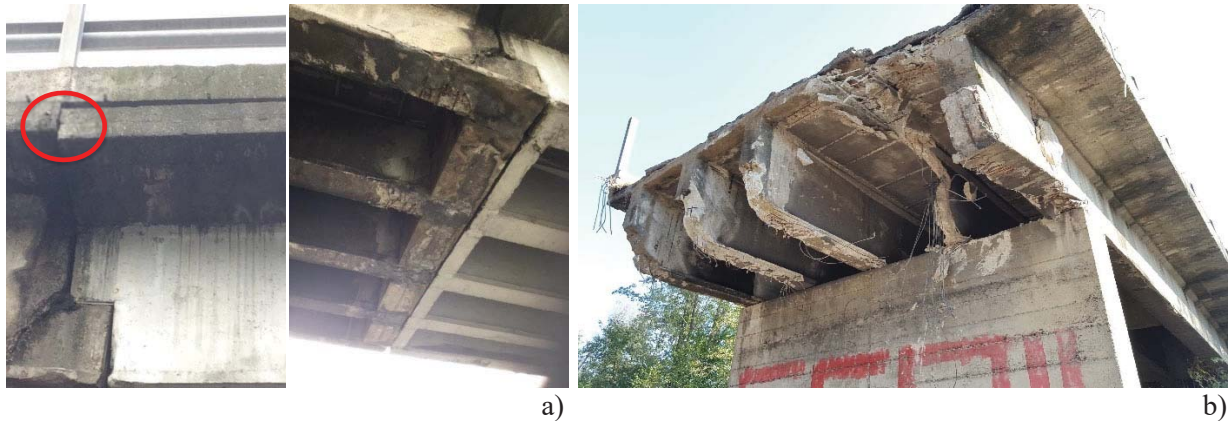
Figure 8-10 – View of the Annone overpass: a) before the collapse; b) after the collapse (di Prisco et al., 2018)
