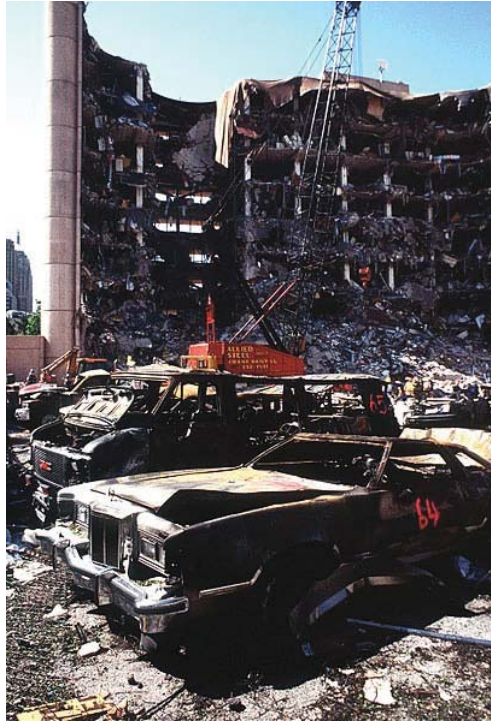
Figure 6-3 – Close-up view of the building after the collapse (from https://commons.wikimedia.org/wiki/File:Oklahomacitybombing-DF-ST-98-01356.jpg )
