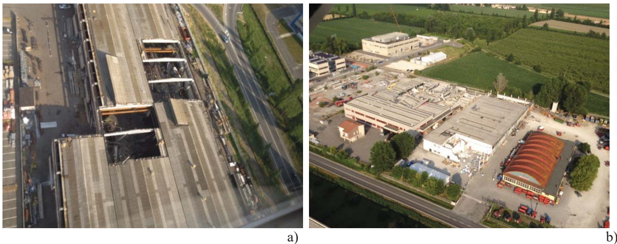
Figure 6-16 – Collapses of precast roof elements often occurred in 2012 Emilia earthquake where irregularities in the building structure were present: a) collapse of roof elements due to plan irregularities; b) collapse of a portion of a two-floor prefabricated building (left) and of lateral spans of another building due to the interaction with masonry infills (right)
