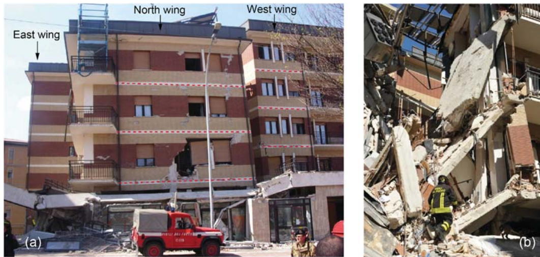
Figure 6-6 – Student house before the demolition of the collapsed wing: a) soft story mechanism in the North Wing; b) Collapse of the columns at the connection between the North Wing (right) and the other wings of the building (left). (adapted from Mulas and Martinelli, 2017)
