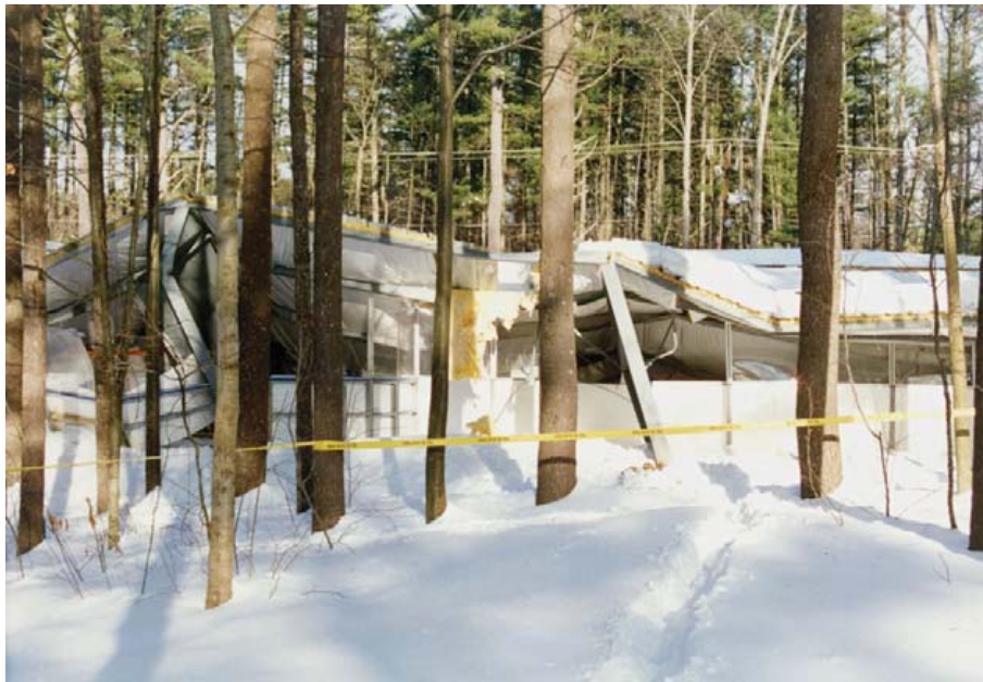
Figure 6-33 – Failure of the roofing of the Jackson Landing Skating Rink (Ellingwood et al., 2007)
