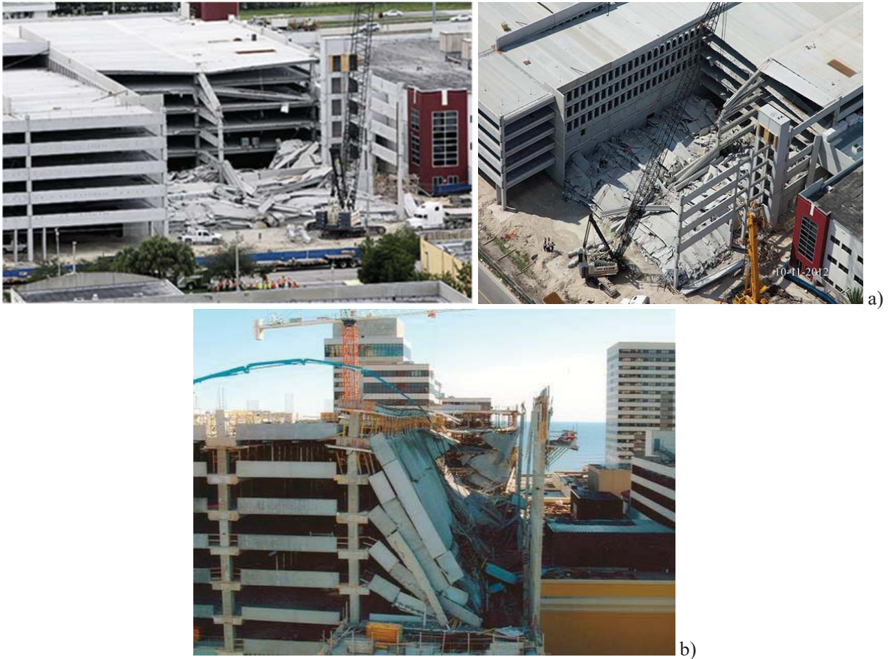
Figure 6-23 – Progressive and disproportionate collapse of precast structures during construction: a) in Miami (from www.osha.gov/doc/engineering/2013_r_02.html ); b) in Atlantic City (from https://failures.wikispaces.com/Tropicana+Casino+Parking+Garage )
