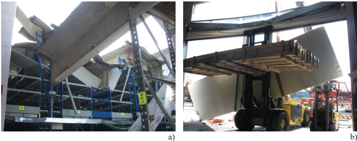
Figure 6-22 – Collapses due to (non seismic) accidental actions: a) collapse due to snow weight which caused high compression stresses and consequent failure of the small dry support of one RC concrete truss beam over the column; b) fall of a RC cladding panel hit by the forks of a mechanical lift during an erroneous operation
