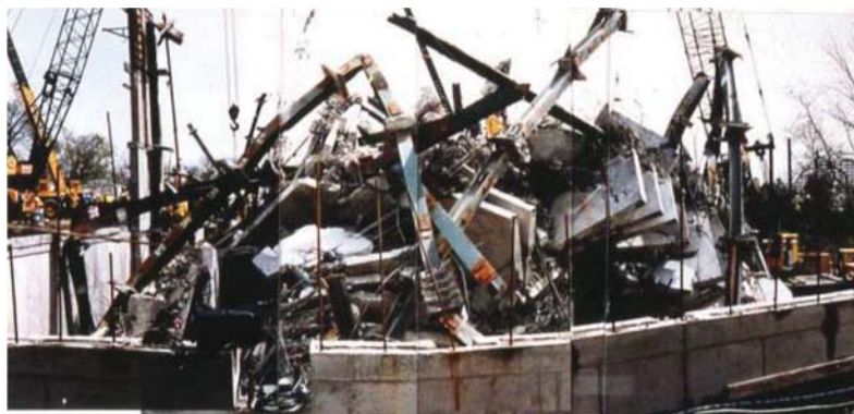
Figure 6-31 – Collapse of the structure of the Ambiance Plaza ( www.bfrl.nist.gov/861/861pubs/collapse/workshop/7.L'AmbiancePlazaCaseStudy060913.pdf )
